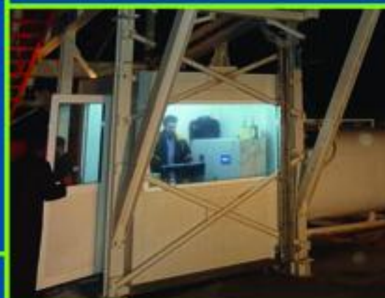
Air conditioned control cabin
